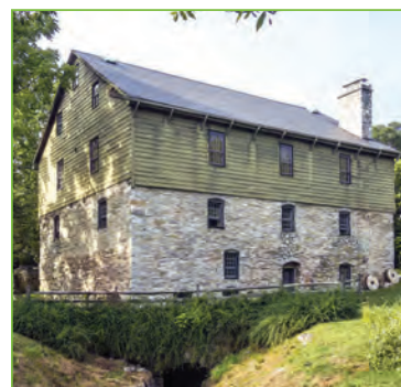
Millwood's Burwell-Morgan Mill, a GCV restoration site. Photo by Calder Loth, courtesy of the Virginia Department of Historic Resources
